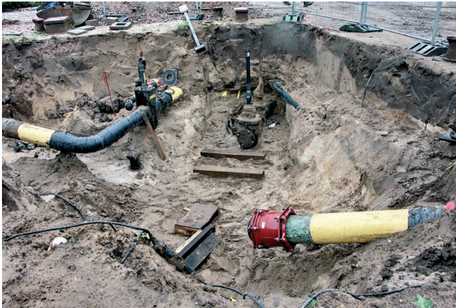
Fig. 4: Small-bore piping on the new gas-pressure regulation system
